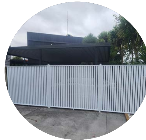
Horizontal & Vertical Panel
